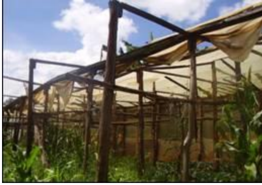
Fig. 1.a: Wrong material for construction
