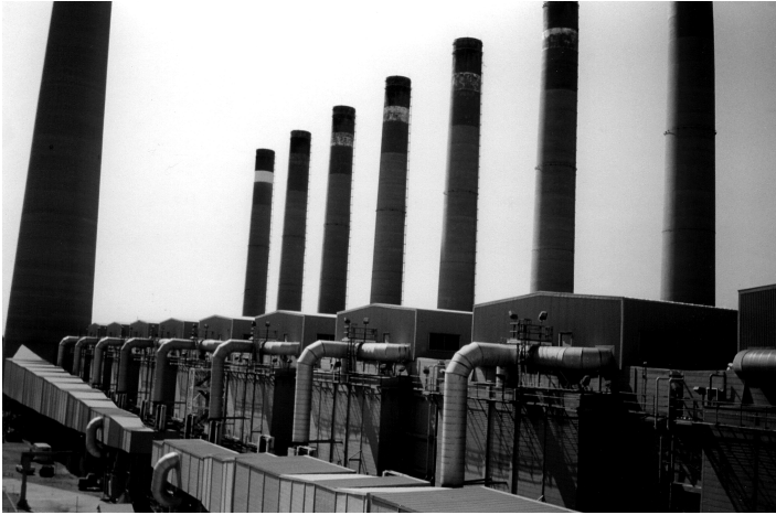
FIGURE 23.3 Large reverse air baghouse.
