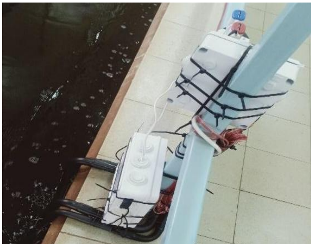
Fig 8: The Central Measurement Node deployed
