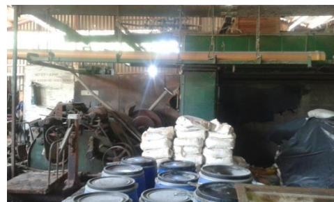
Figure 0.6: Broken down boiler unit. Source: STL
