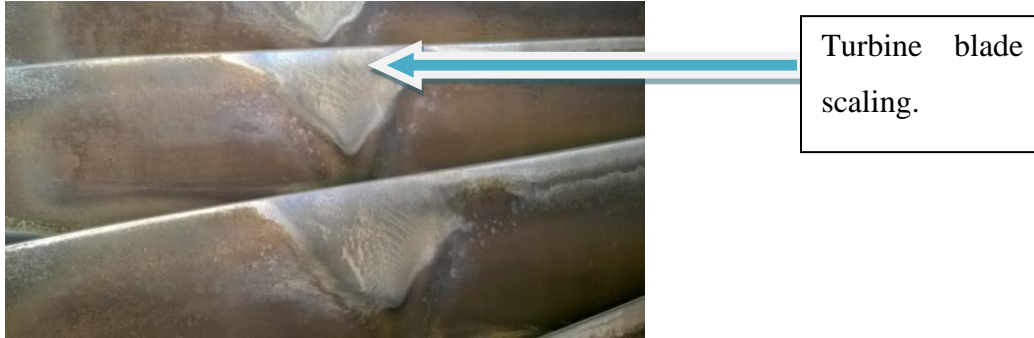
Figure 2. 10: Turbine blade scaling
