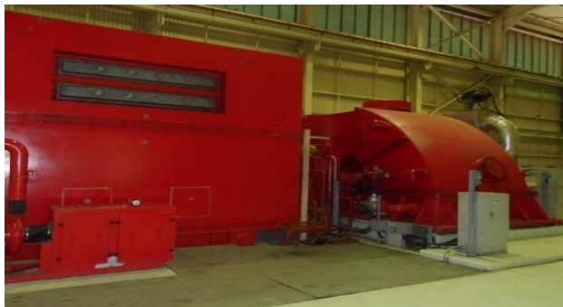
Figure 2. 9: The turbine-generator assembly at Olkaria II power plant
